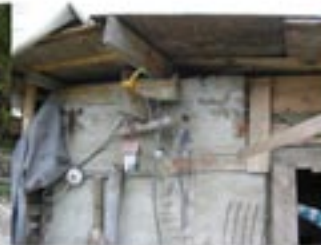
electrical conduits wired into wall
